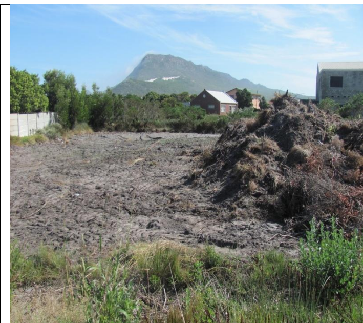
Sharp sticks remaining are removed together with a large amount of topsoil.
